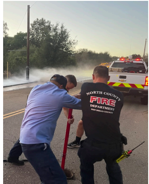
North County Fire Protection District assisted Rainbow Municipal Water District staff with shutting down a fire hydrant.
